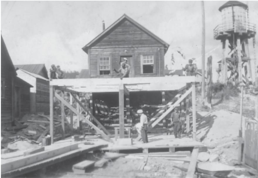
Volunteers building an addition onto the Japanese Hall, Paldi, BC. (Tom I. Tagami photo, 1940)
